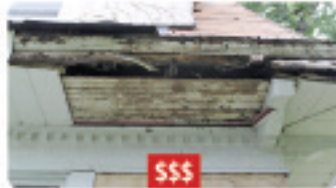
Rotting Fascia & Soffit
