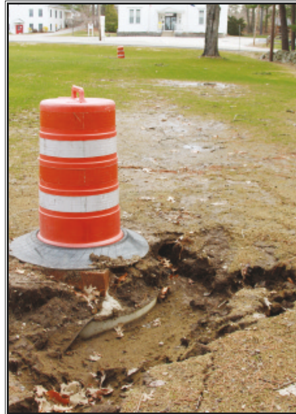
Winter weather took a toll on the drainage work done on the Town Common last fall. Phase II of the project is expected to start soon.
