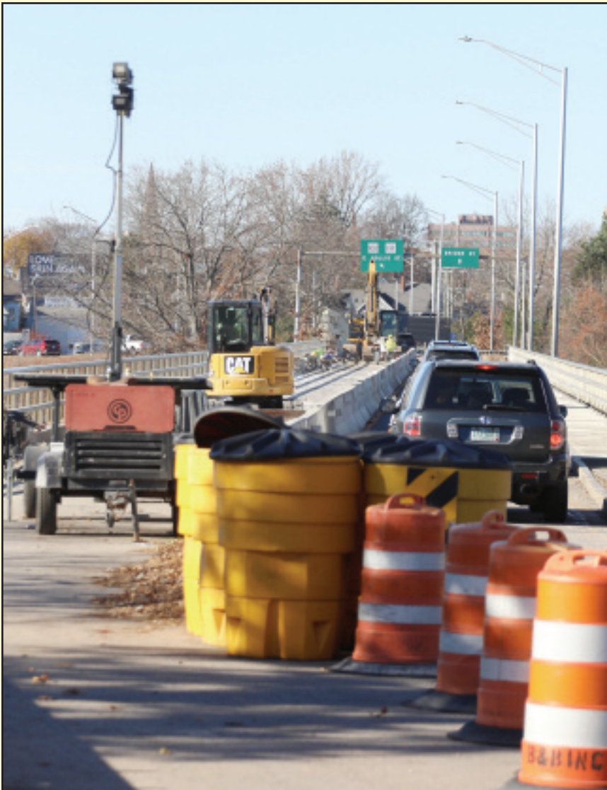
SLOW & STEADY Construction on the right lane of the Veterans Memorial Bridge is complete, leaving the left lane to be finished up. The completion of the project is expected to happen before the end of the year. Workers will move to the Taylor Falls Bridge in April of 2025. Photo by Chris Paul
